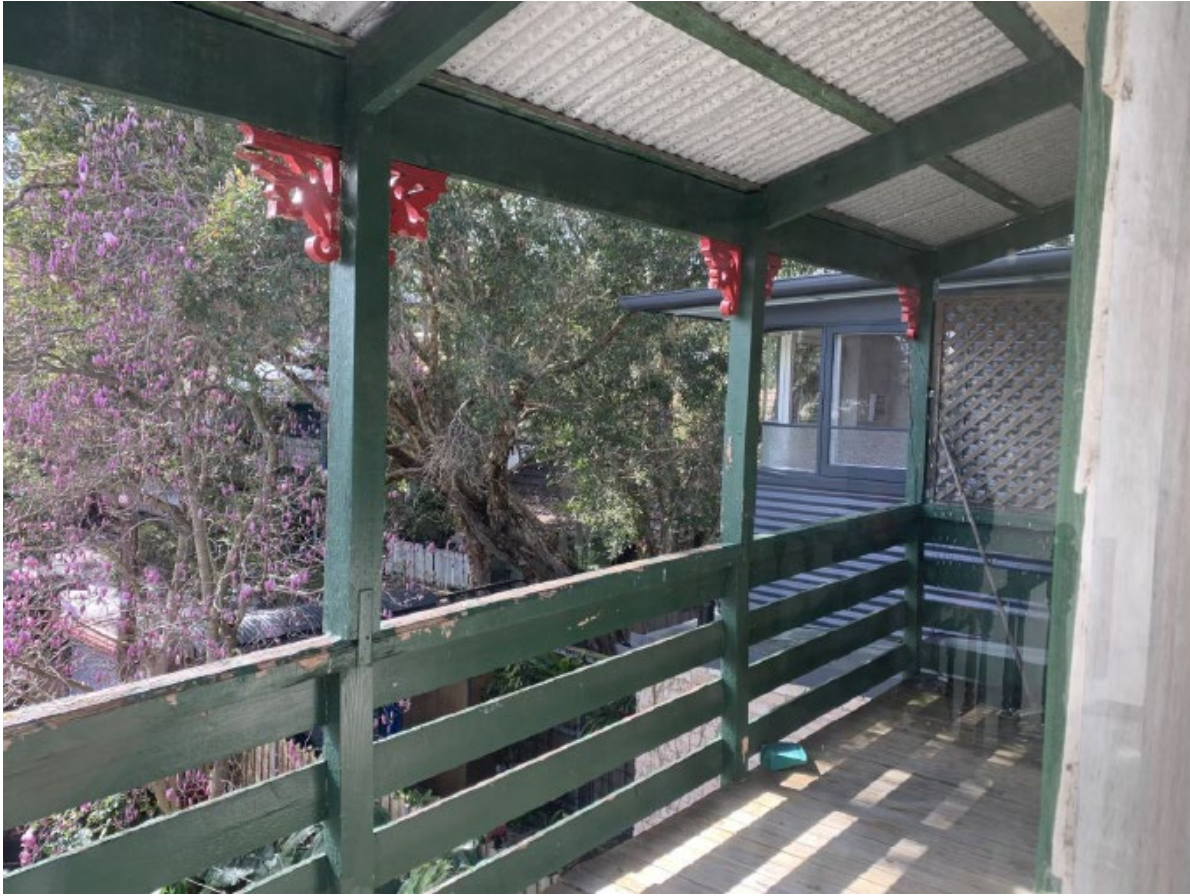
First floor showing the first floor of No. 47 to the east of the subject site
